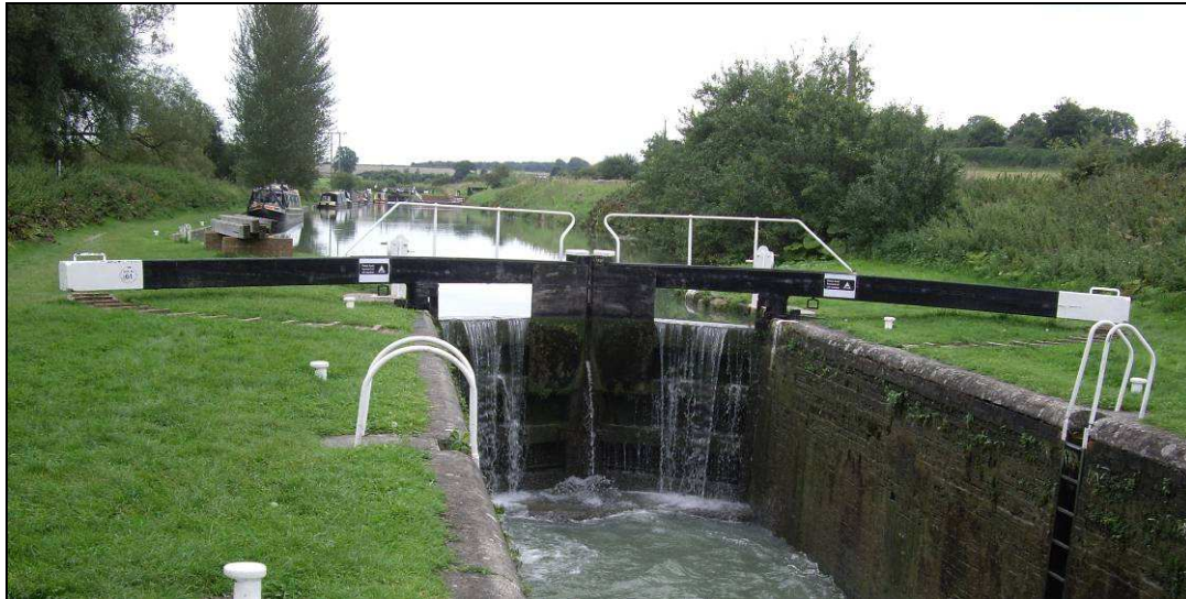
Figure 24. Water overtopping lock gates during a period of high flow.
