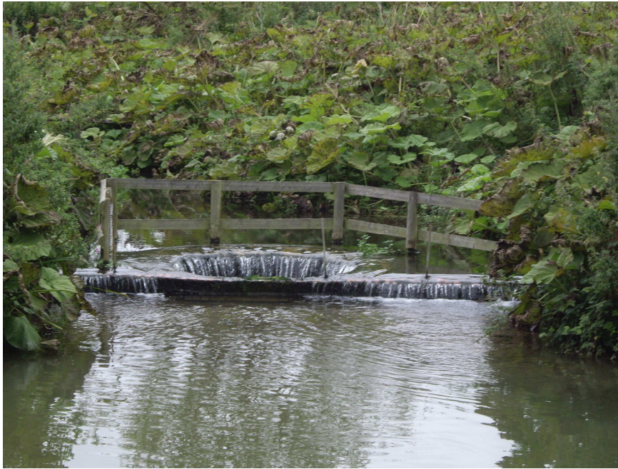
Figure 47. Control structure to divert Froxfield Stream flow away from the canal.
