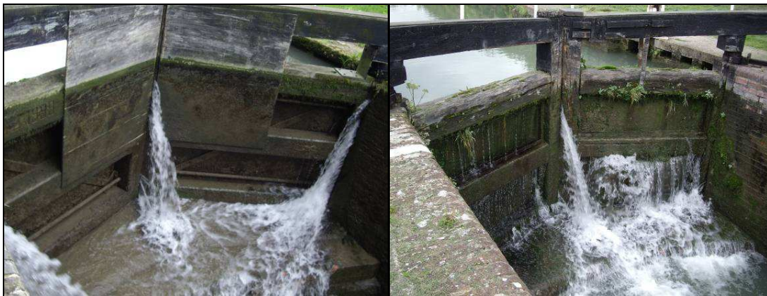
Figure 6. Typical leaking lock gates. Note reinforced center of gates where boats push in the left image.
