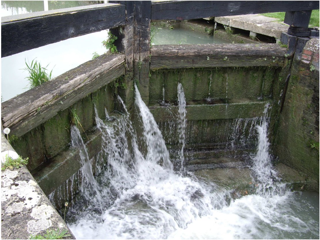
Figure 51. Example of leaky lock gates.
