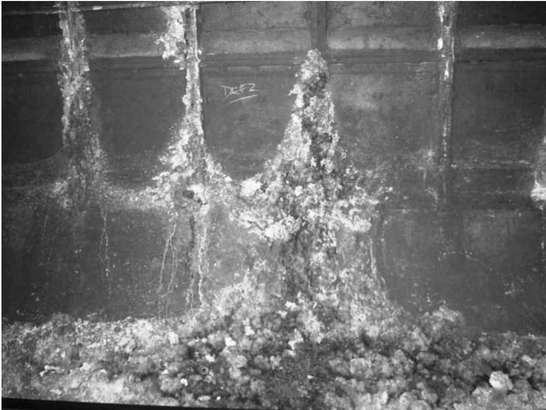
Figure 5.9: Lining deposits in a London underground tunnel
