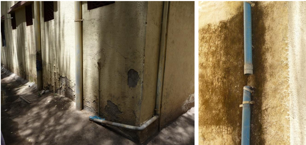
Figure 63 – Failing plaster and down-pipes
