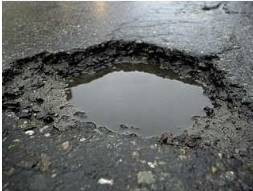
Figure 1.4: Large pothole in road (AA Ireland website, 2011).
