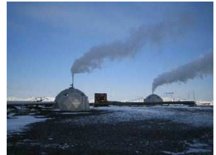
Figure 25.11. More geothermal power in Iceland. Photo by Rosie Ward.
