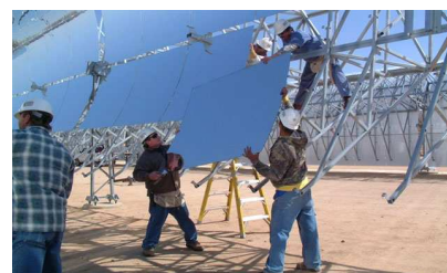
Figure 25.4. Andasol – a “100 MW” solar power station under construction in Spain. Excess thermal energy produced during the day will be stored in liquid salt tanks for up to seven hours, allowing a continuous and stable supply of electric power to the grid. The power station is predicted to produce 350 GWh per year (40 MW). The parabolic troughs occupy 400 hectares, so the power per unit land area will be 10 \text{ W/m}^2 . Upper photo: ABB. Lower photo: IEA SolarPACES.
