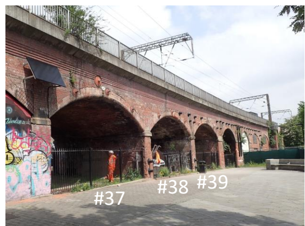
Figure 2. The southern side view of the Marsh Lane Viaduct in Leeds, UK
