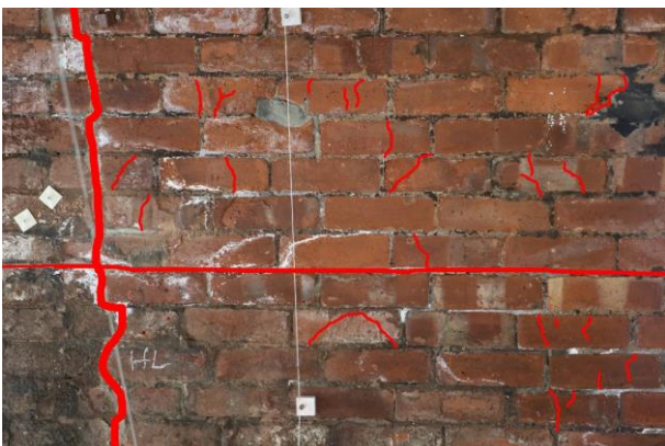
Figure 9. Cracks observed near sensor 37NA7A8
