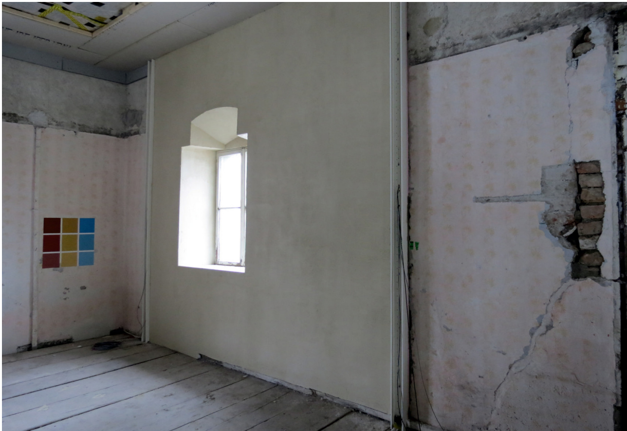
Figure 2 An overview of the room, containing a test field that has had the complete insulation system applied (central area, between the cable trunking, and including the window). To either side of the test field, the original historic wall surface is visible. Photo: Fraunhofer IBP.
