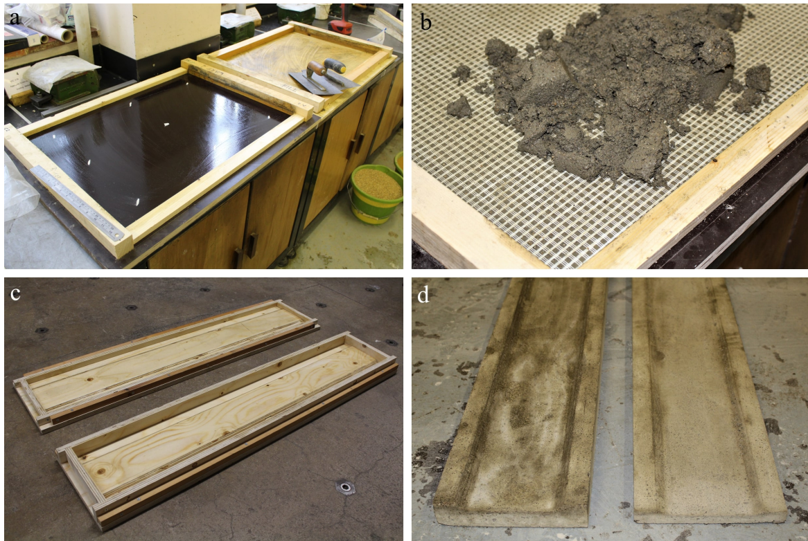
Figure 4.6: Construction of TRC test specimens, showing a) panel formwork for tensile and bending specimens, b) fine-grained concrete prior to trowelling, c) compression specimen formwork and d) de-moulded compression specimens prior to cutting.
