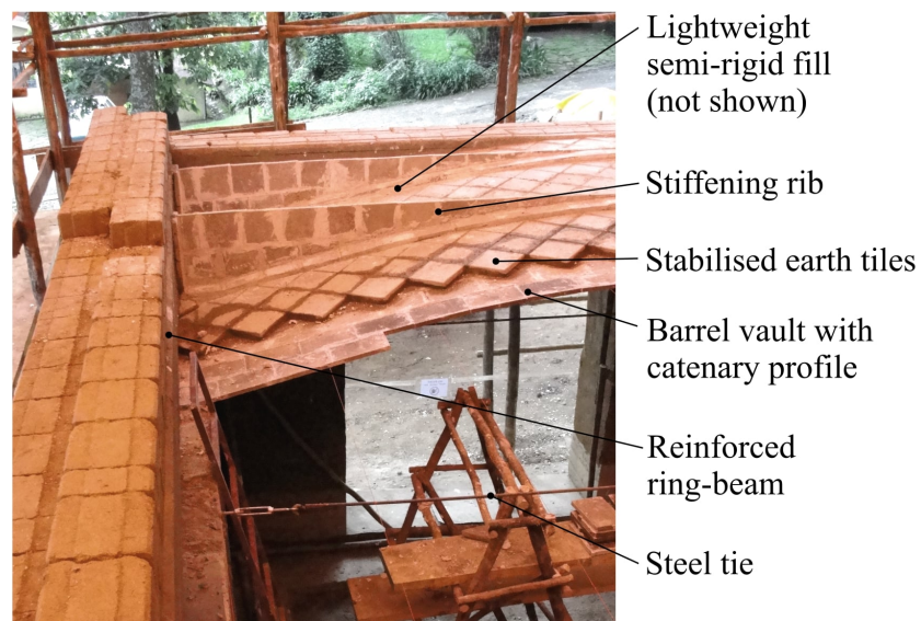
Figure 2.11: Tile barrel vaulted floor with stiffening ribs (photo Lara Davis, with permission).
