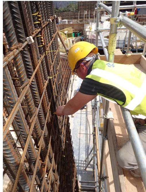
Figure 4 The fibre optic sensing cables being attached to the reinforcement of column C8 before being concreted.
