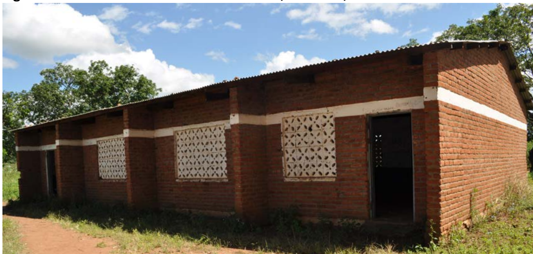
Figure 9.1: Disused double classroom block, School B, Zone 9
